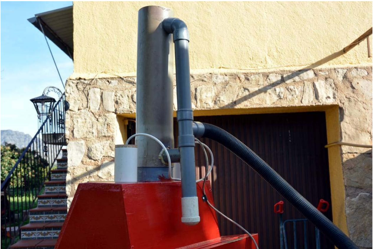
Showing the large diameter tower with the smaller diameter down tube and shopvac connection. There is a short connecting tube near the bottom of the tower, this is a structural support for the down tube.
