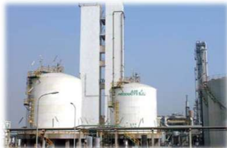
Figure 2 Cryogenic air separation plant with heat exchanger and distillation column towers
